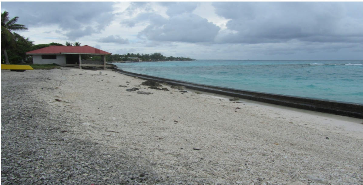
Figure 6: A bulkhead on the lagoon side of Avatoru, with beach erosion still unprevented. Image: Anna Rios Wilks (Dec, 2012).
